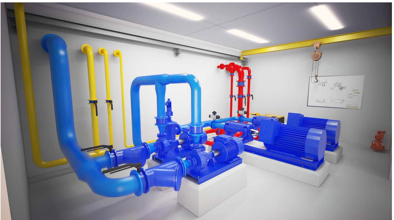
Pump station with preliminary pressure and high pressure pump
